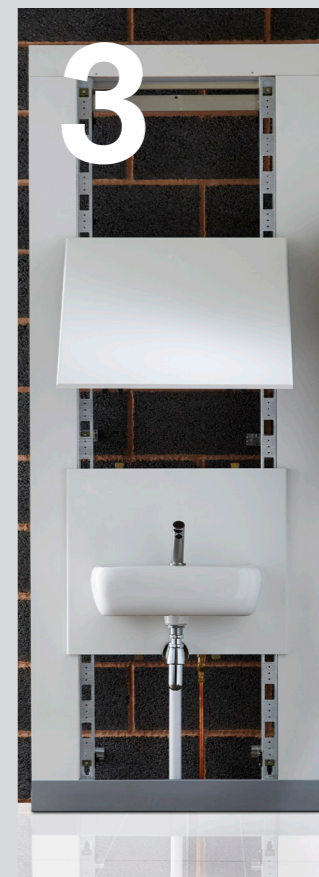
03 Once all the units are in position, connect the plumbing and services.
